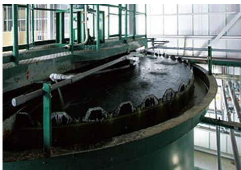
Waste-water treatment plant
